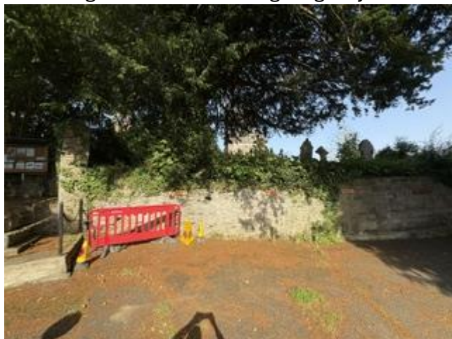
Retaining wall cracked and giving way
